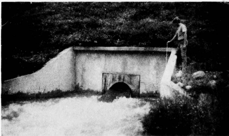
M. Outlet Works During Operation of Slide Gate.
