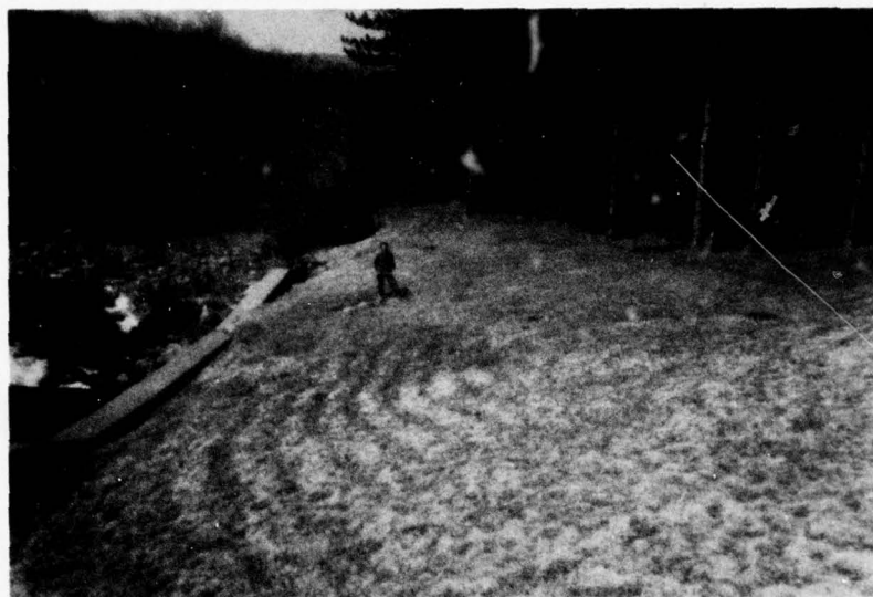
E. Area Adjacent to Embankment Damaged by Surface Runoff
