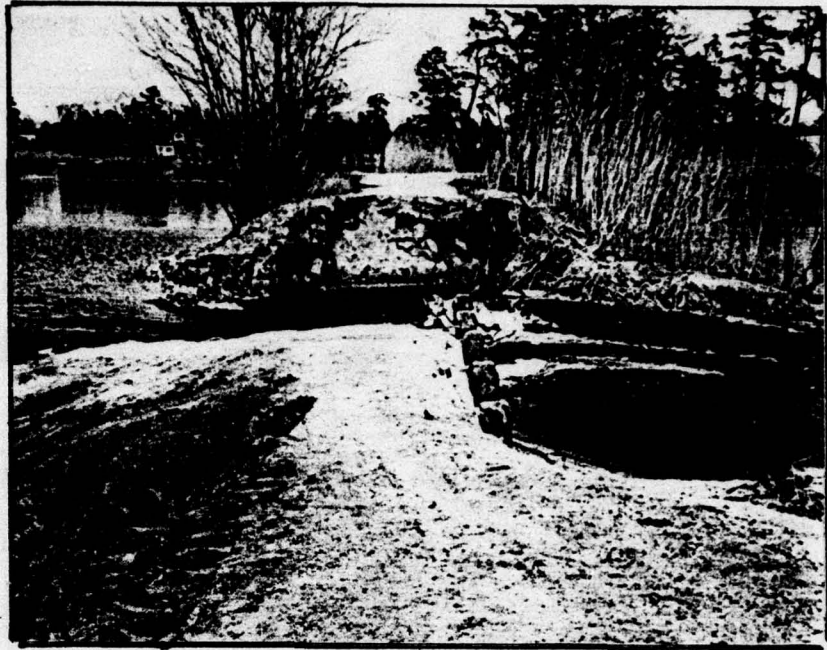
Upstream dam failure
