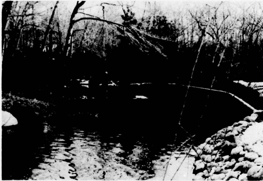
Photo 8 - Concrete weir at end of lined channel downstream of the spillway. (November 30, 1978)
