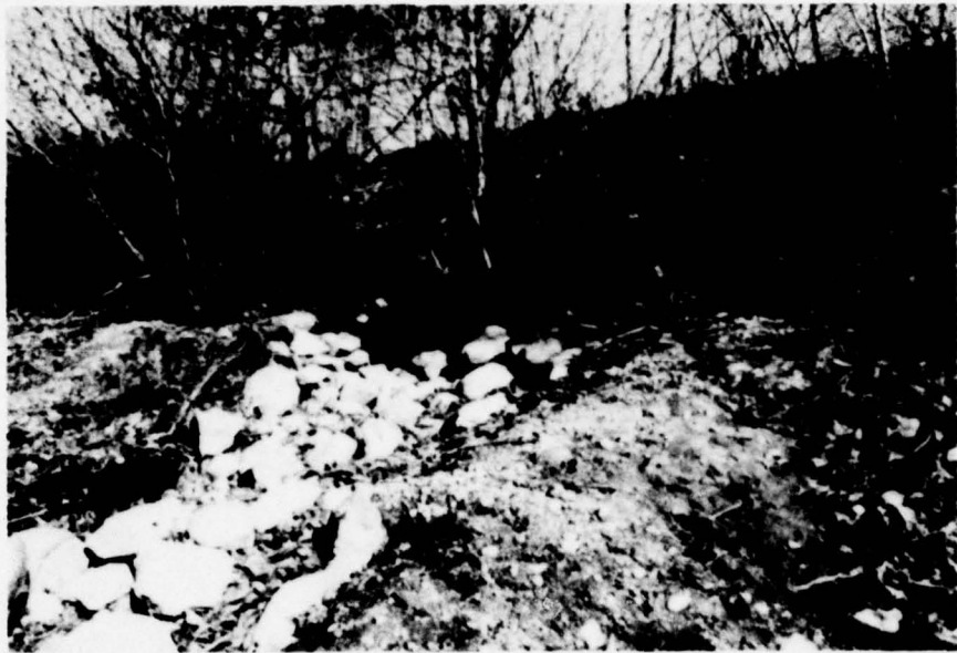
Photo 3 View of stone filled gully in central section of the downstream face of embankment
