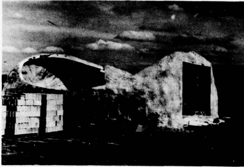
Figure 16. Collapsed arch 5 weeks after completion.
