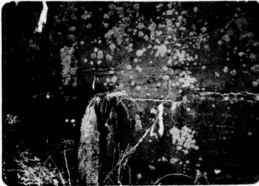
Water leaking through face of dam at right side of spillway.
