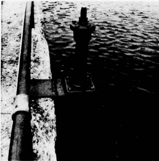
OPERATING MECHANISM OF SLUICE GATE
