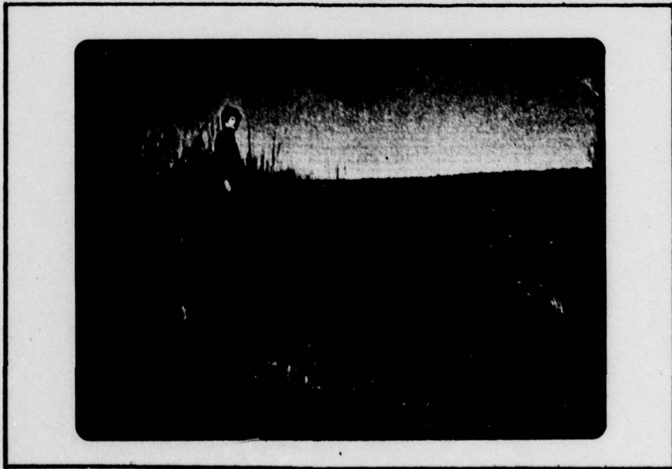
UPSTREAM FACE OF THE DAM SHOWING THE OVERGROWN BRUSH
