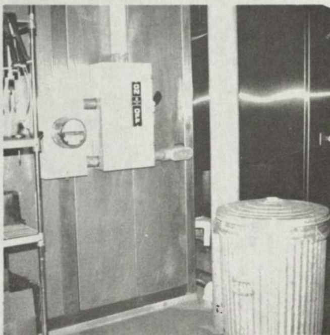
Fig. 3. Electric Meter for Measuring Electricity Consumption of Revolving Tray Oven at CFPF.
