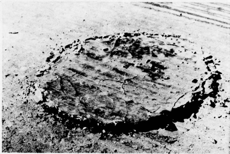
Figure 53. Small Crater Polyester Repair Did Not Bond to Edges
