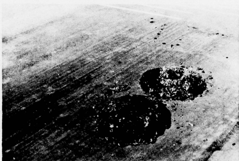
Figure 54. Small Crater Repair Removed
