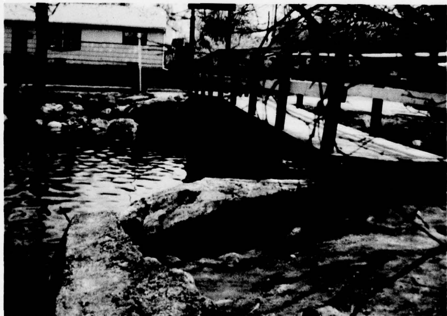
PHOTO 2 DETERIORATION OF CONCRETE AT SPILLWAY
