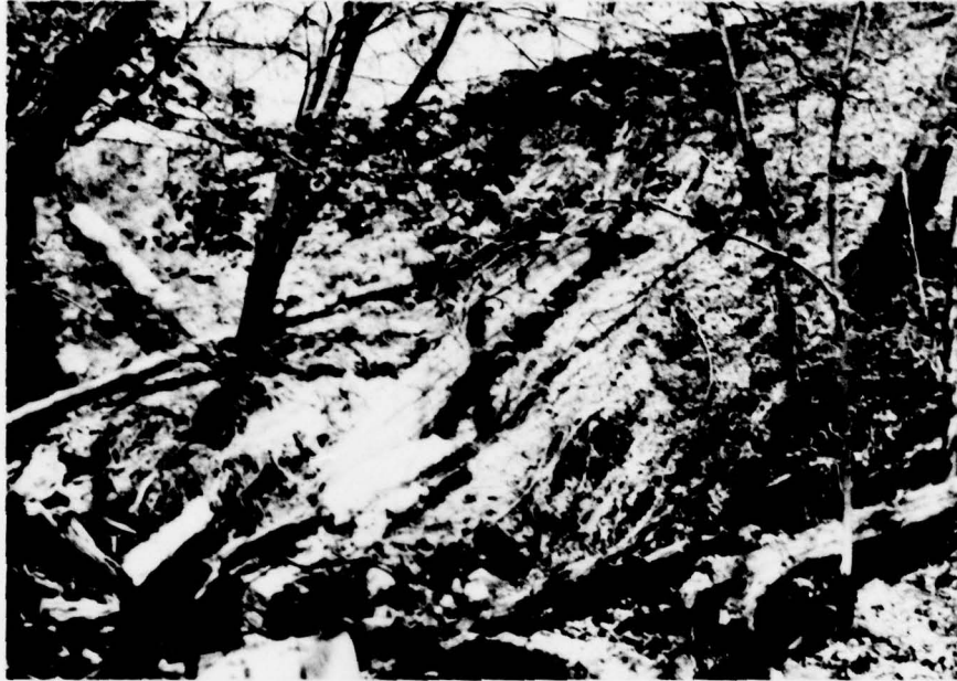
Photo No. 3 - View of left downstream face near spillway showing severely eroded embankment slope and fallen trees. Note also the retaining wall at toe.
