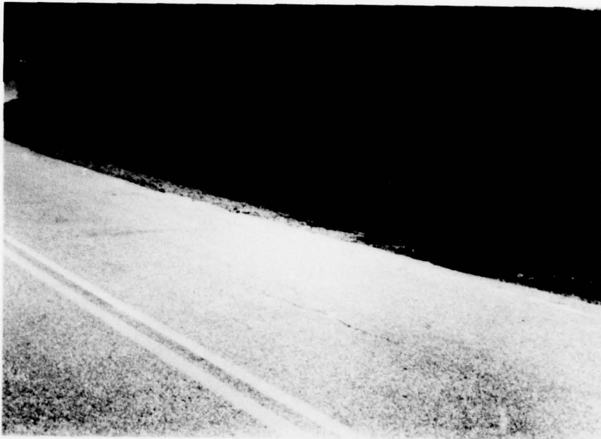
Photo No. 3 - View of Pleasant Valley Road looking to the right. Note the crack in the pavement and the trees on the upstream slope of the embankment.
