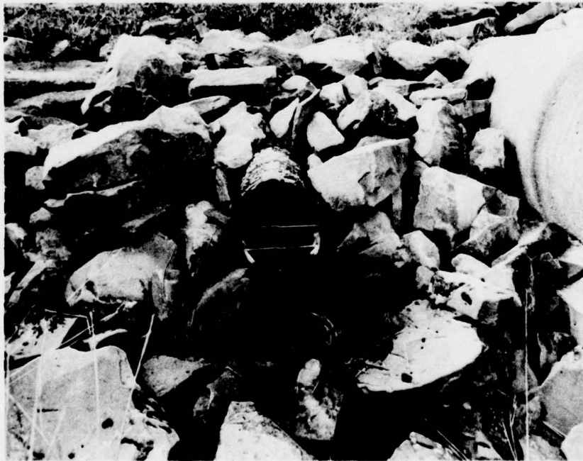
OUTLET OF INTERNAL DRAINAGE SYSTEM COLLECTION PIPE
