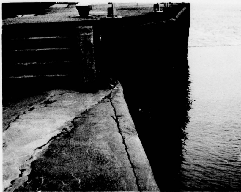
CONCRETE SURFACE DETERIORATION @ LOCK - SPILLWAY CONTACT
