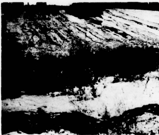
Figure 16. Overall view of damage incurred by water main break, looking southeast.
