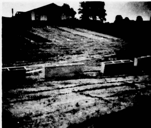
Figure 18. View of finished plots prior to the installation of the sediment tanks.
