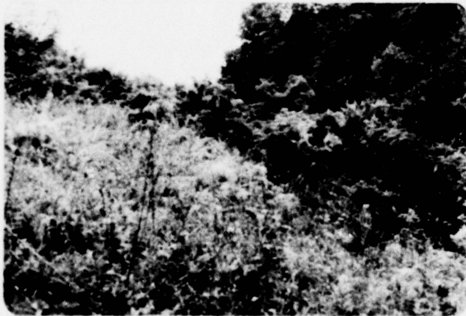
PHOTO * 6 HEAVY VEGETATIVE GROWTH ON DOWNSTREAM SLOPE
