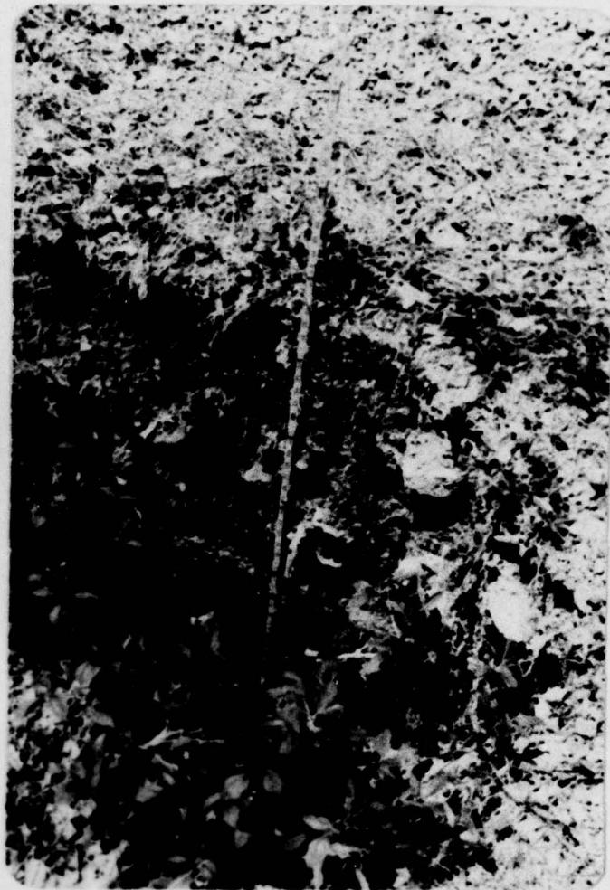
PHOTO # 7 EROSION AROUND DOWNSTREAM END OF EMERGENCY SPILLWAY
