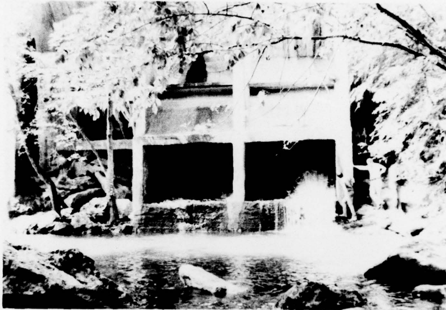
PHOTOGRAPH NO. 5 Discharge from Slide Gate
