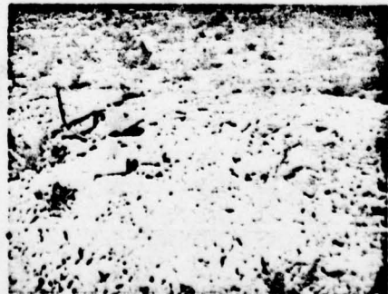
TIPPED OVER—PARAPET PARTIALLY LEVELED.
