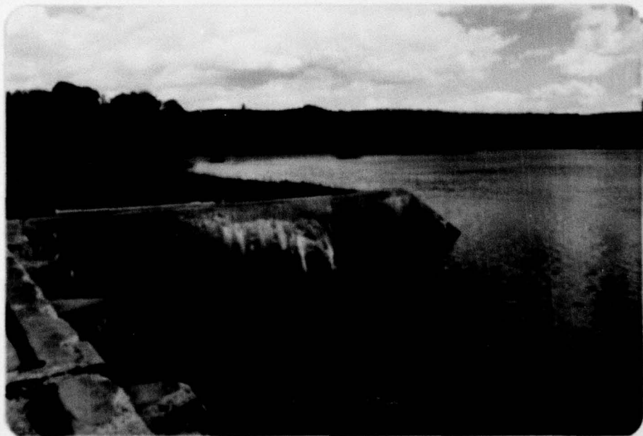
Deterioration of Concrete on Wingwall on East End of Spillway
