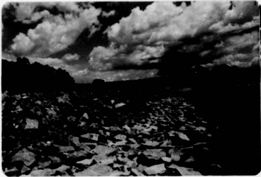
Riprap on Western End of Dam - Gray Stone Placed Due to Damage by Wave Action
