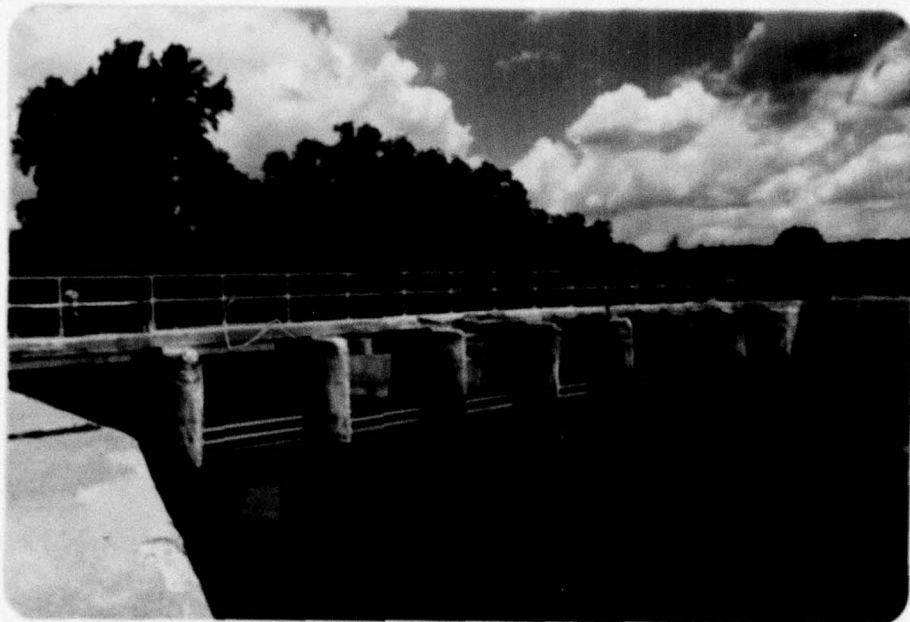
Spillway Section - Channel Stopgates in Place
