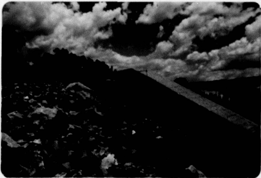
Depression on West End of Spillway Caused by Wave Action
