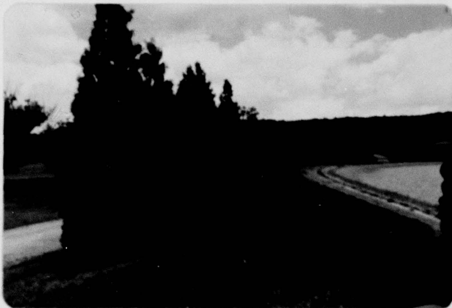
Trees Growing on Downstream Slope at Eastern End of Dam
