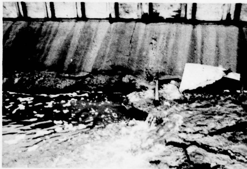
EROSION OF BEDROCK @ SPILLWAY
