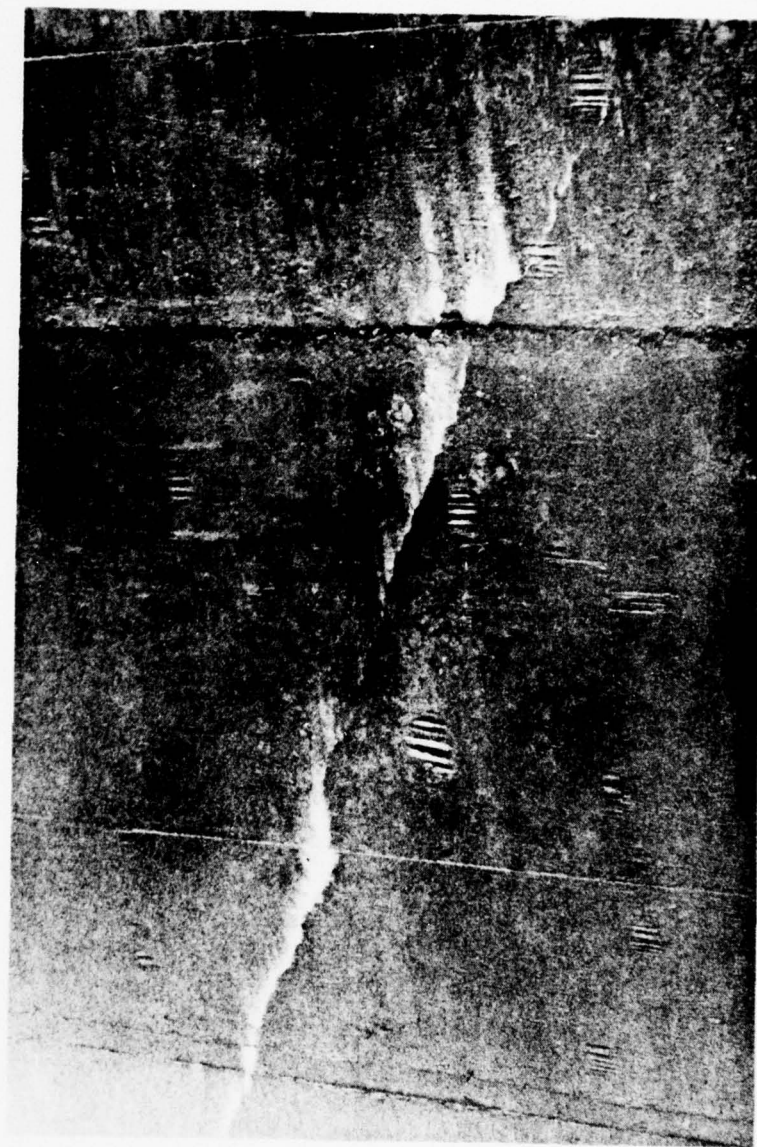
CRACK IN SURFACE
