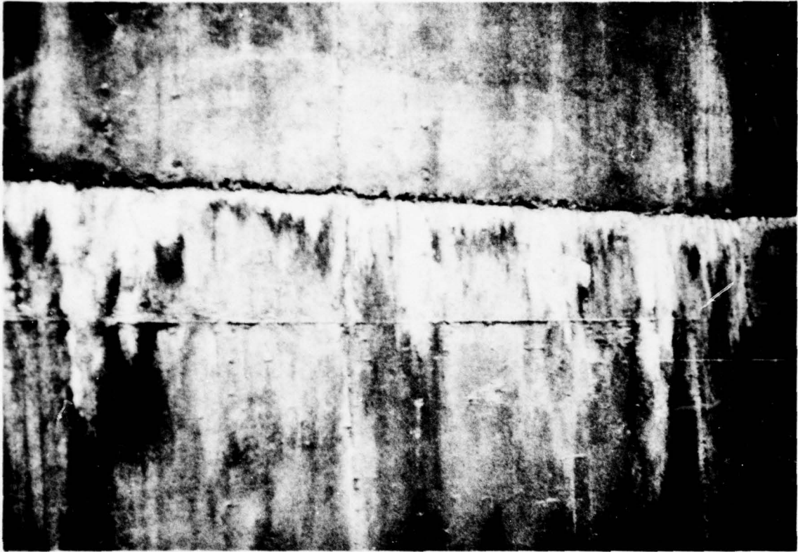
VIEW OF COLD JOINT
