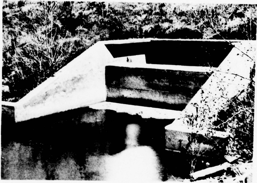
OUTLET ENERGY DISSIPATOR Note: Outlet Channel Flow
