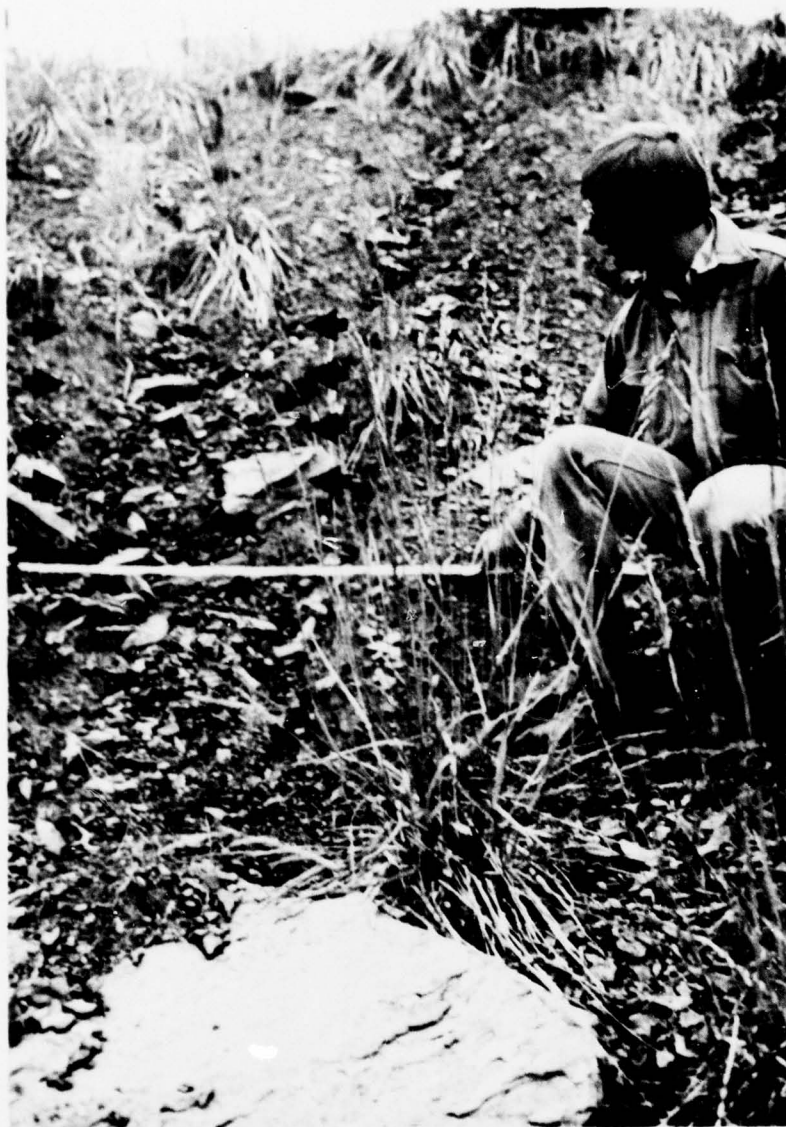
EROSION ON DOWNSTREAM FACE
