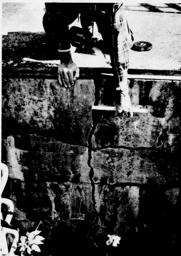
Figure 7. Cracked lock wall, Oliver Lock, Tuscaloosa, Alabama
