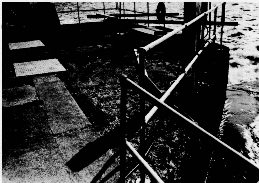
Figure 1. Deteriorated surface concrete, Troy Lock and Dam, Hudson River, Troy, New York
