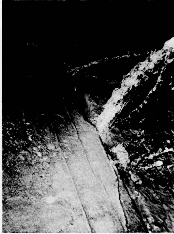
b. Leakage through construction joint in entrance shaft to dam tunnel
