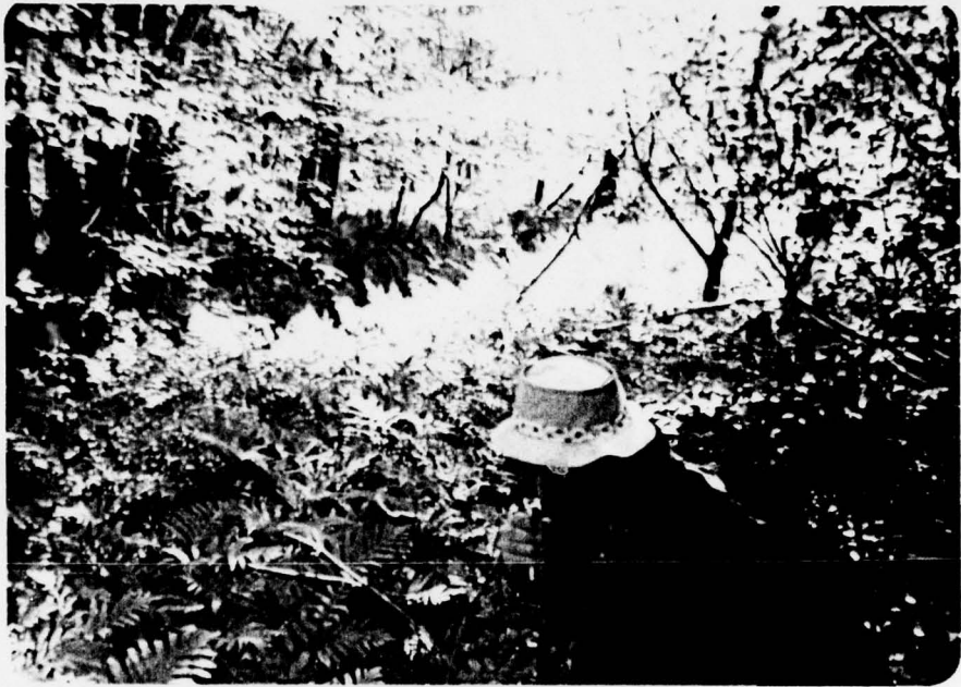
8. Wet area along drainage ditch at toe of embankment on west portion of dam.
