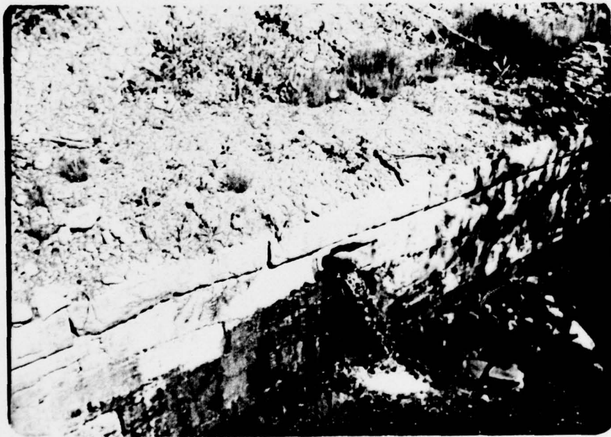
11. Substantial flow from west side of dam drainage system.
