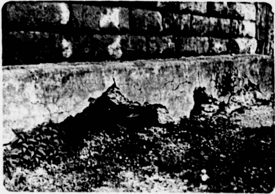
12. Undermining of Oneida Street Bridge pier adjacent to downstream gate of lock.
