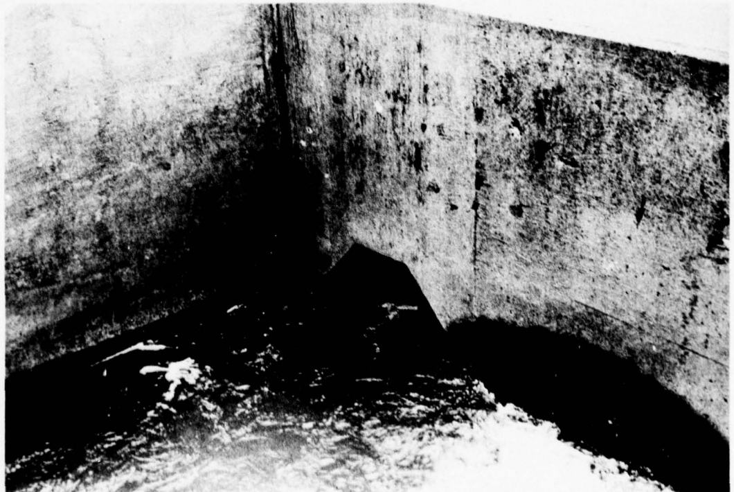
PHOTO 4. Concrete Surface and Opening in Baffle Wall of Impact Basin
