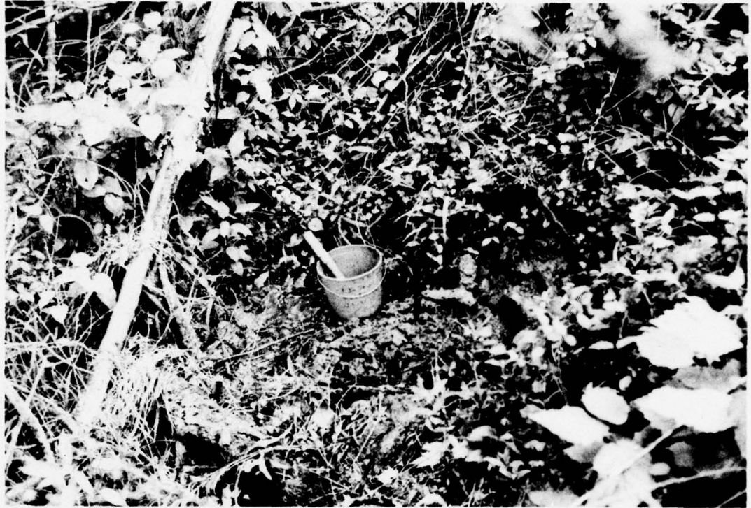
PHOTO 3. Close-up View of Seepage Area Located Near Right Side of Outlet Pipe
