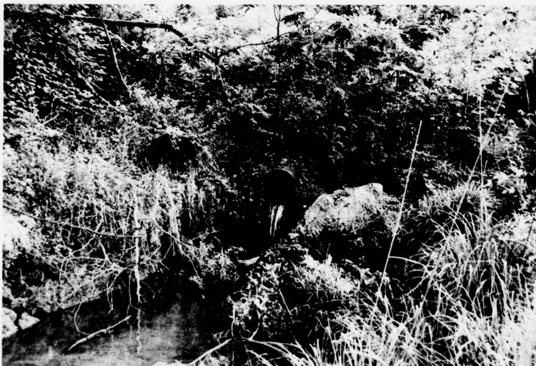
PHOTO 6. Outlet Pipe and Debris in Stilling Basin
