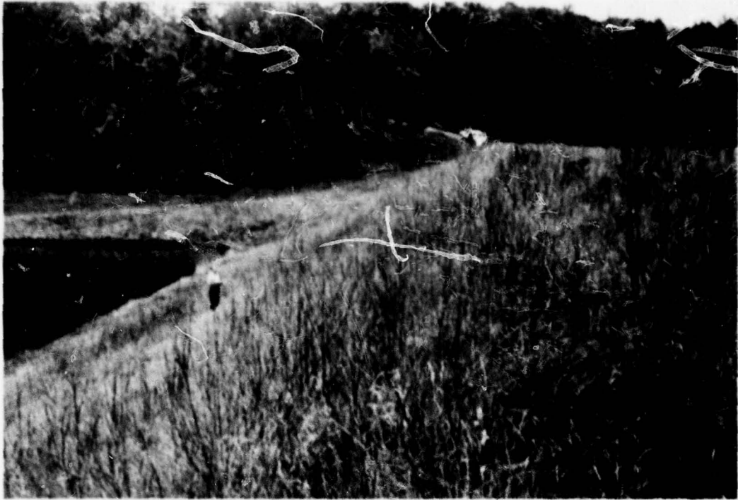
PHOTO 1. Upstream Face of Dam Showing Tall Weeds in Grass
