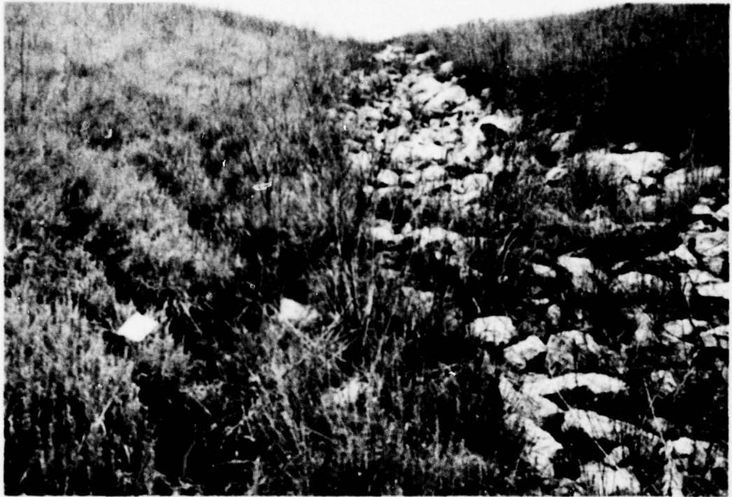
PHOTO 3. Junction of Dam and Right Abutment (Upstream Slope) Showing Erosion Gullies Adjacent to Rock Slope Drain
