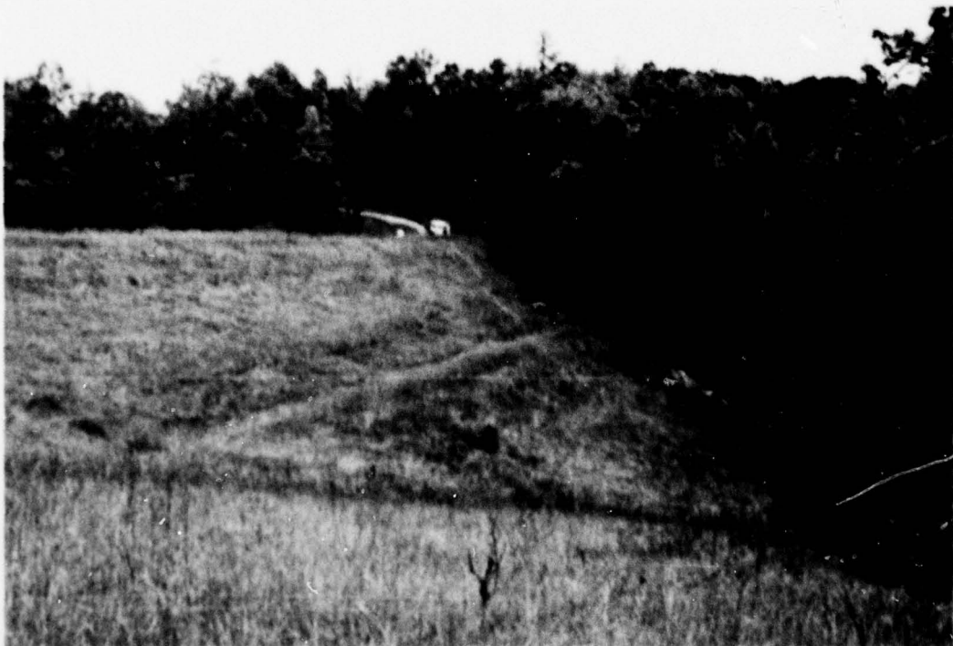
PHOTO 2. Downstream Face of Dam Showing Tall Weeds and Bench
