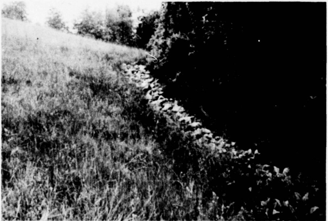
PHOTO 4. Junction of Dam and Left Abutment with Rock Drain on Downstream Slope
