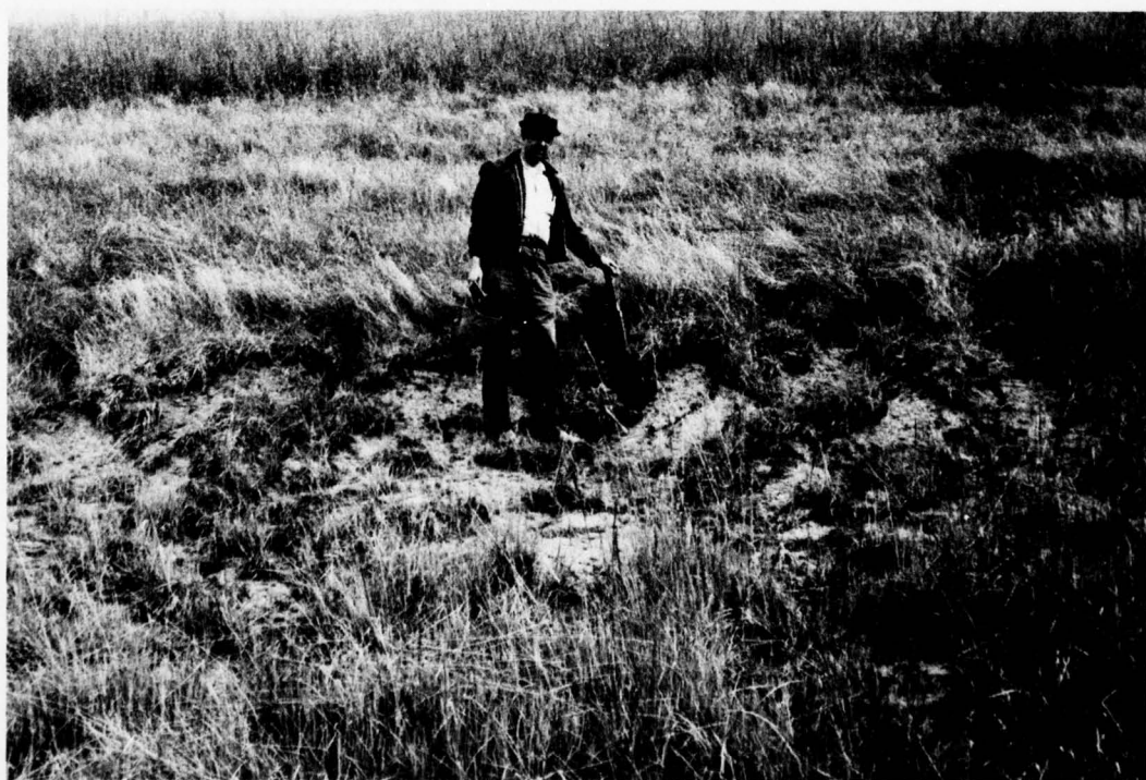
PHOTO 2. Sloughing and Erosion Area Near Upstream Left Abutment
