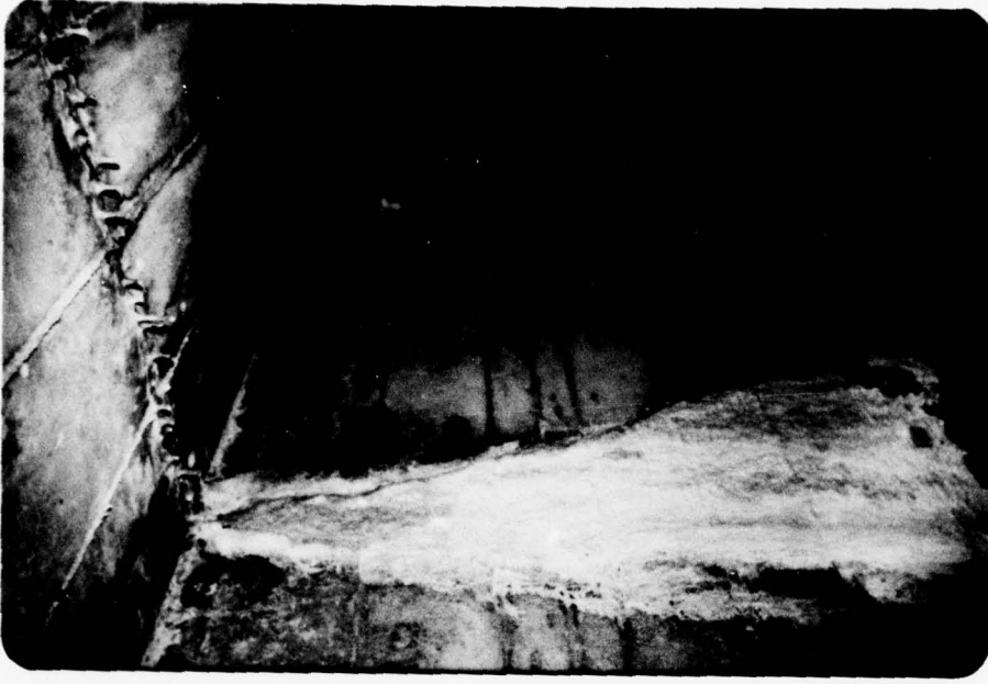
Reservoir Drain Interior Note Calcification at Construction Joint Photo #9
