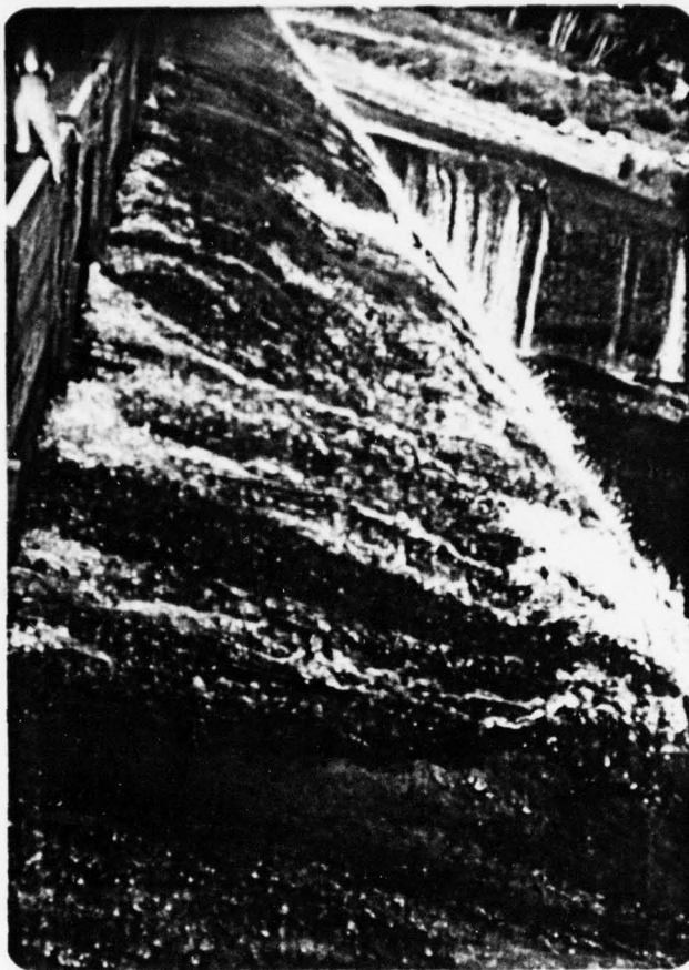
5. Close-up of eroded spillway surface near the north abutment of the south dam section.
