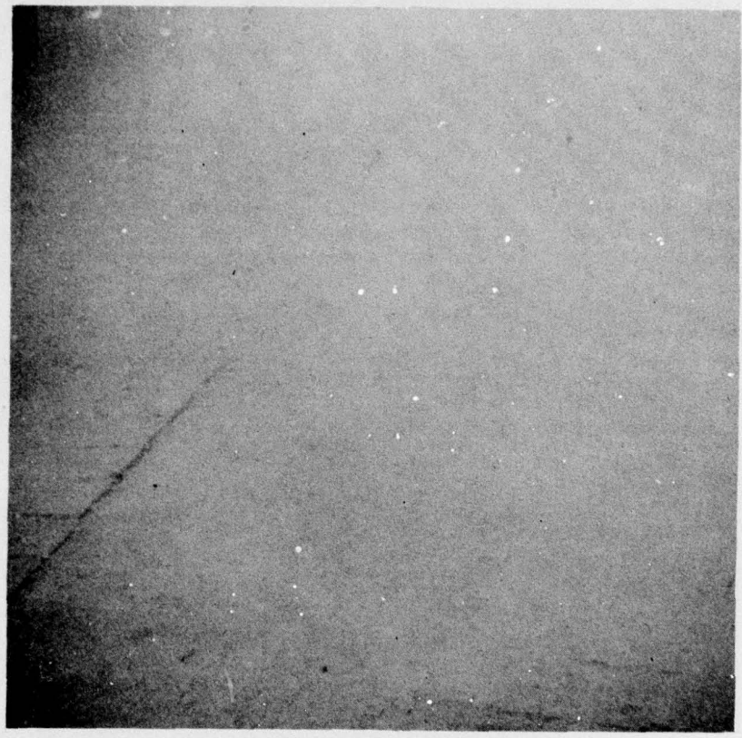
Damaged wood decking in way of top forward end of stack. ABCR Photo No. 6007-6.
