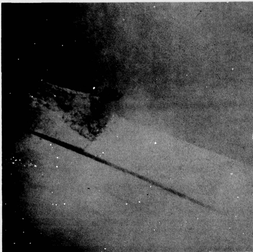
Damaged wood decking in way of broken stanchion, starboard side, between 5" 38 cal. mount #5 and forward deck house, about frame 59. ABCR Photo No. 6005-8.
