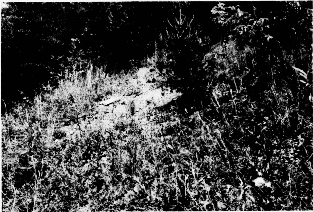
PHOTO 7. Small Slumps in Hillside Cut of Right Emergency Spillway
