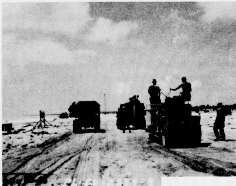
Watering and rolling the cement-coral sand mix in the soil stabilization operations, Aomon-Bijiri.
