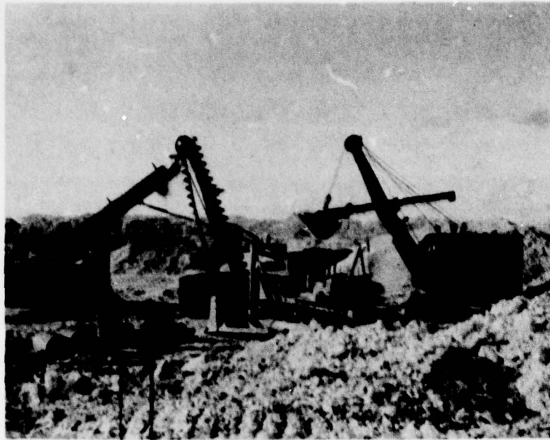
Coral Rock Crushing Operations on Engebi, 20 January 1948. The crushed coral was used for making the concrete used for instrument buildings
