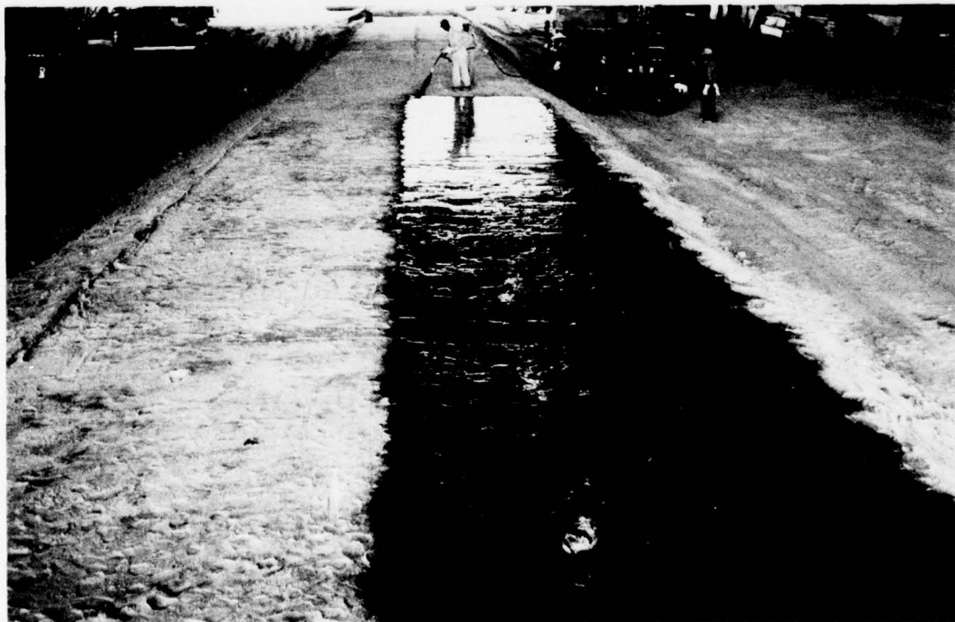
Photo 14. Spraying RC 800 liquid asphalt on sand surfacing, east half of test section, test section 1
