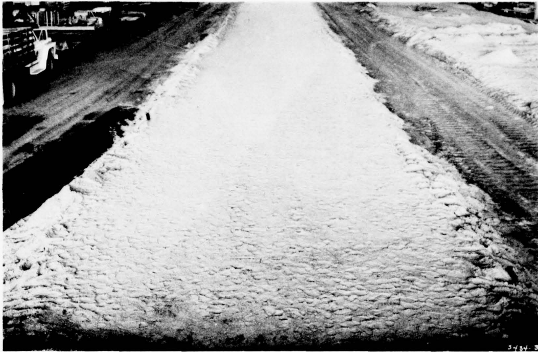
Photo 1. Base layer of sand on which test items were constructed, test section 1
