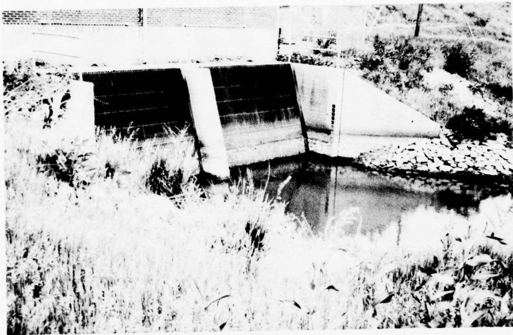
Figure 11. Entrance to sump, 45-deg wing walls, rounded pier noses, pumps not operating
