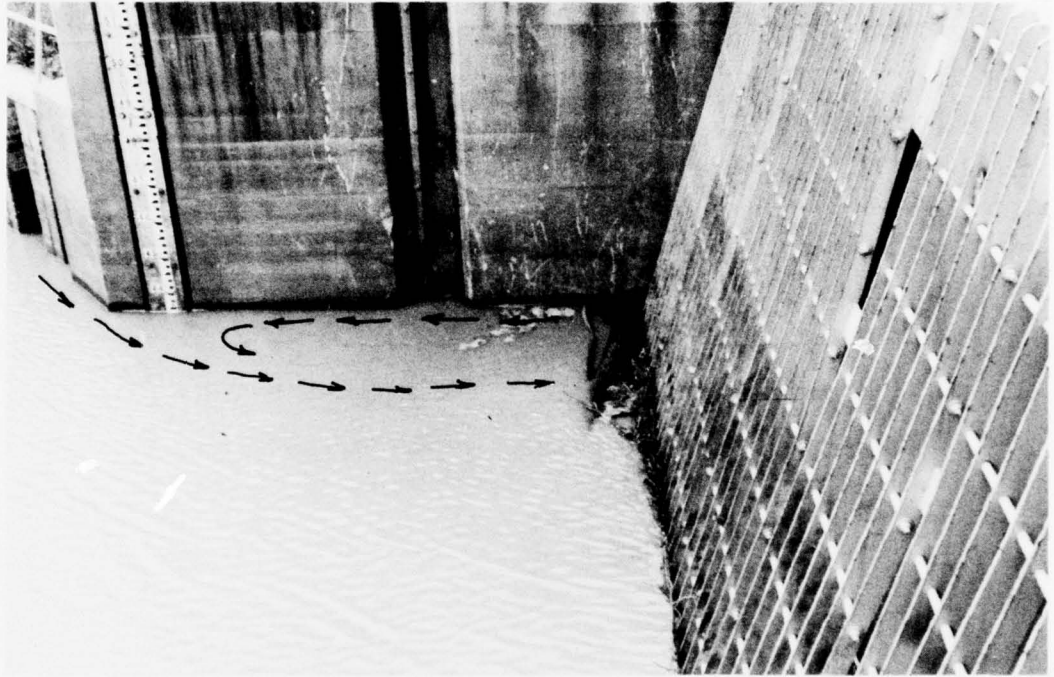
Figure 17. Entrance to sump, 45-deg wing wall, adverse circulation
