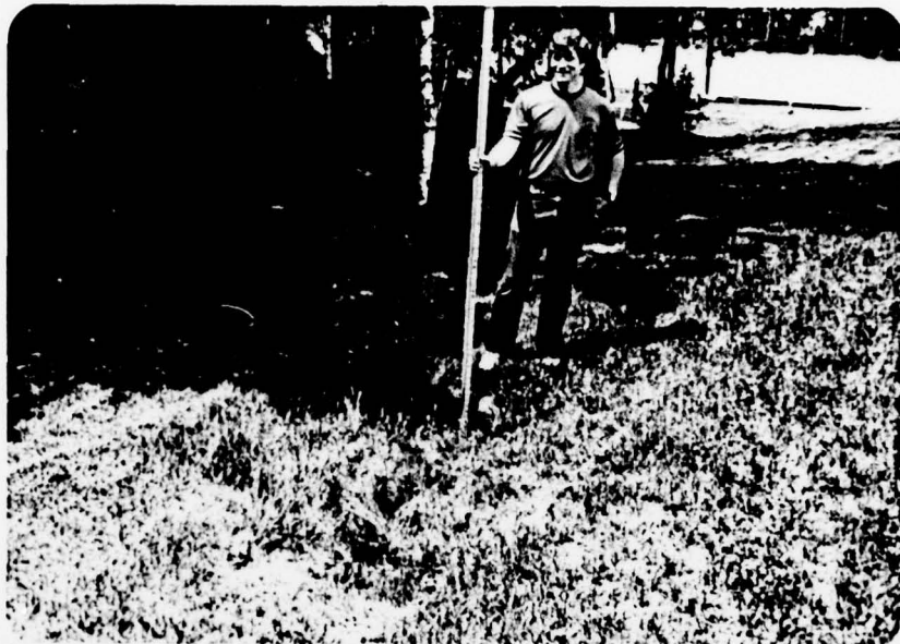
C. Burrowing Animal and Stump Hole in Embankment
