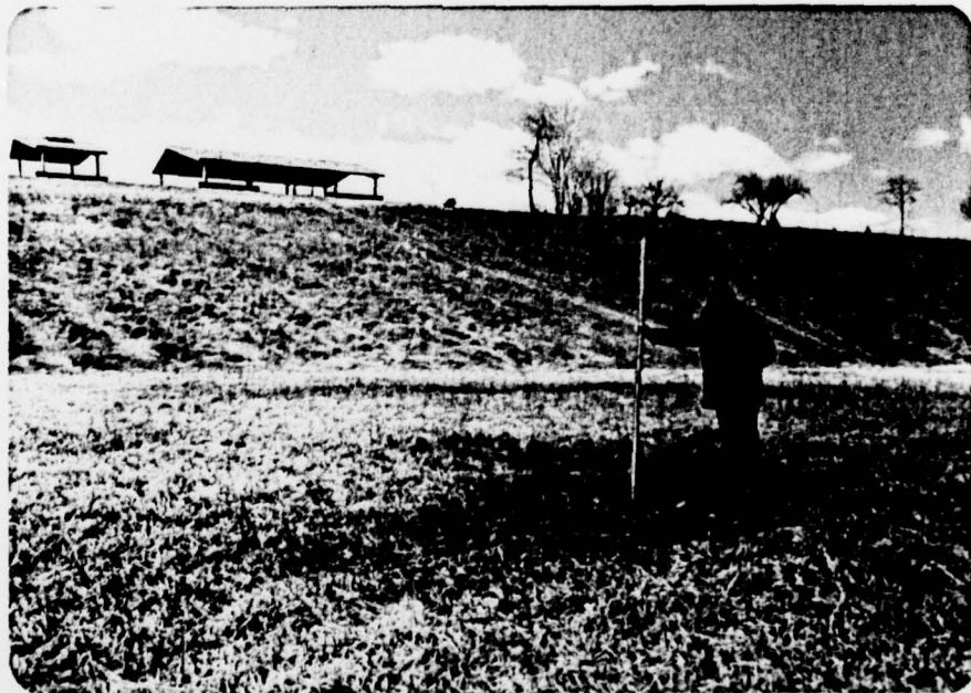
H. Sinkhole in Auxiliary Spillway
