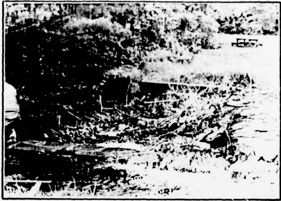
Debris blocking spillway.
