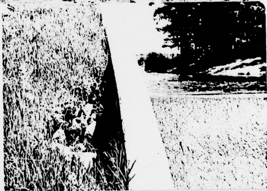
Settlement Adjacent to Right Spillway Wall
