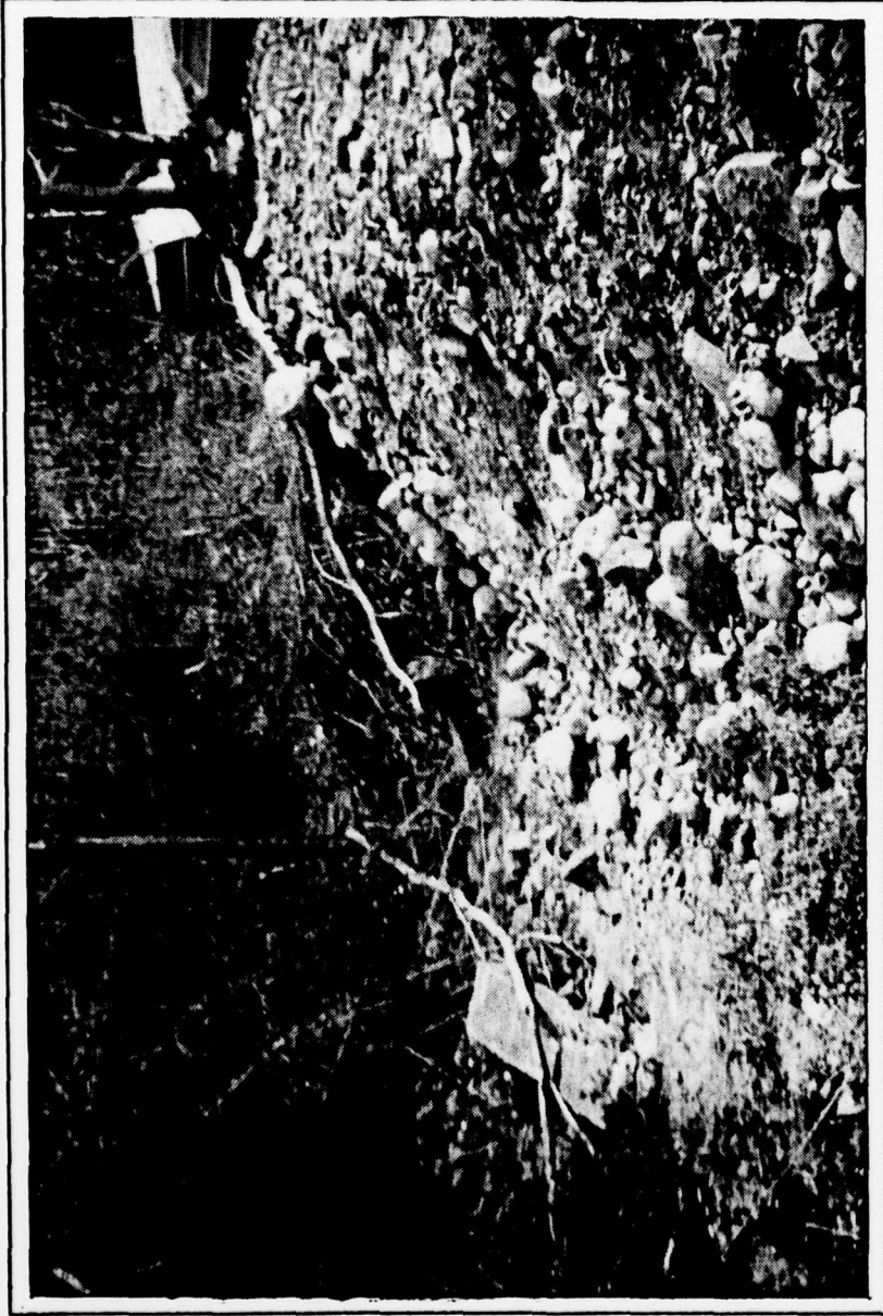
AREA DOWNSTREAM OF AUXILIARY SPILLWAY SHOWN IN PHOTOGRAPH NO. 12. NOTE THAT FILL WAS NOT COMPACTED OR FOUNDATION PREPARED.
