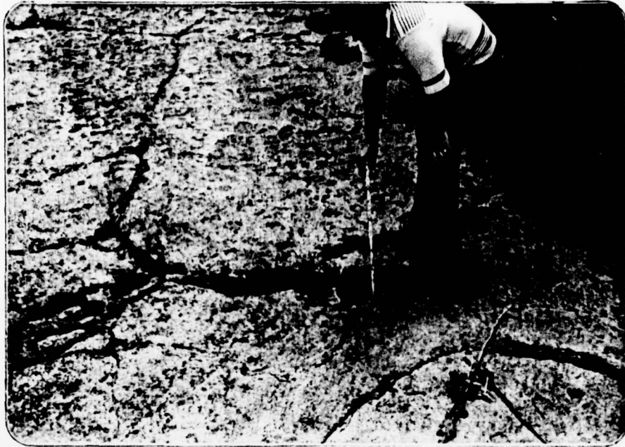
PHOTO 9. Close-up View of Cracking and Loss of Material Beneath Spillway Slab
