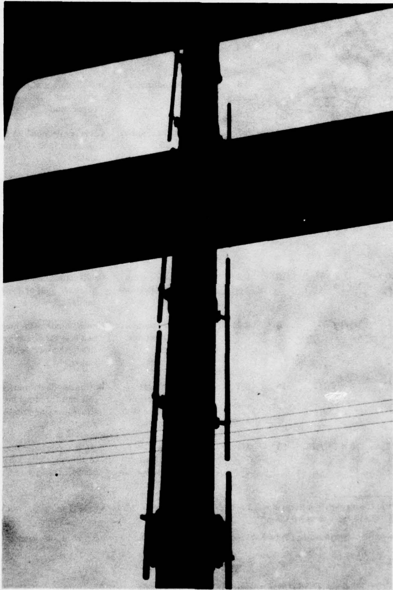
Figure 4. Cathodic protection by sacrificial magnesium anodes of intake gates in Portland District (Dalles Lock and Dam).
