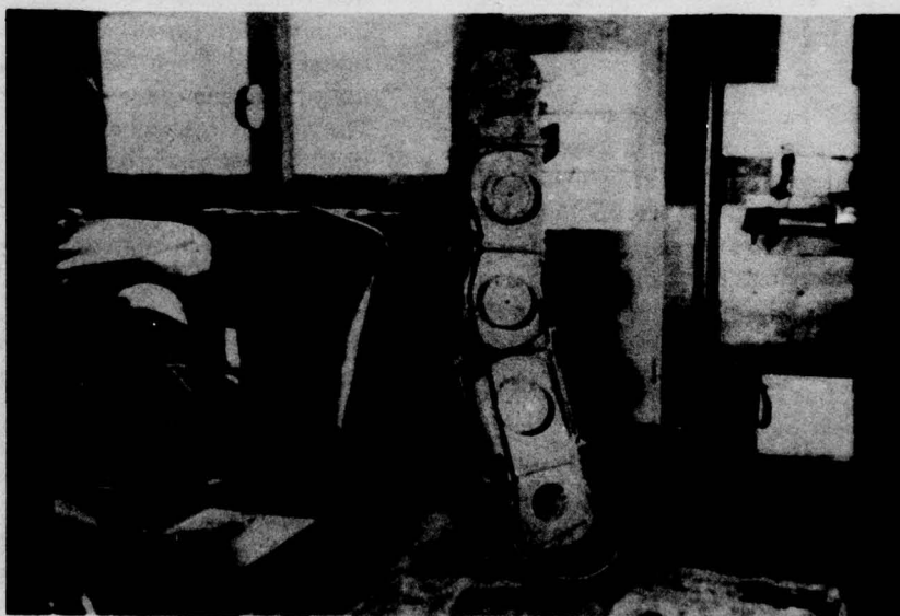
Figure 27. Experimental cathodic protection of tainter gate raising chains at Rock Island District.
