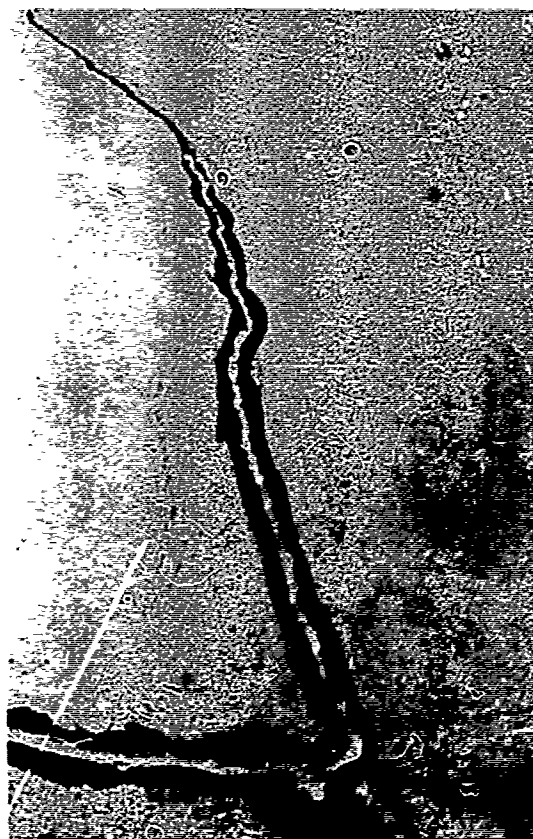
Photo 99. Crack No. 12 on northeast corner of wall.
