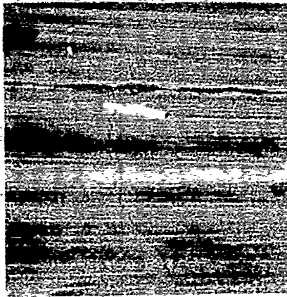
Photograph 1. Crack No. 1 on runway location prior to sealing. This was a very narrow, hairline-type crack.
