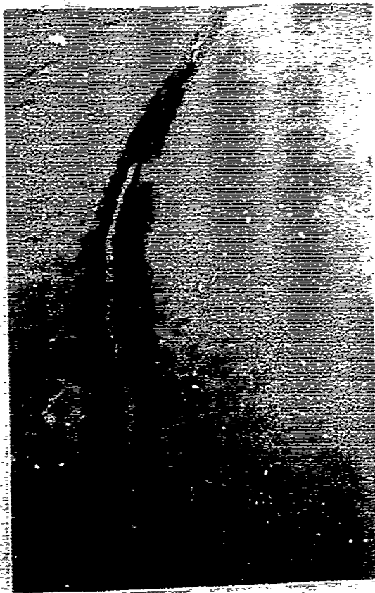
Photograph 26. Coast Pro- Sent in crack No. 16 on northeast walk-up apron.
