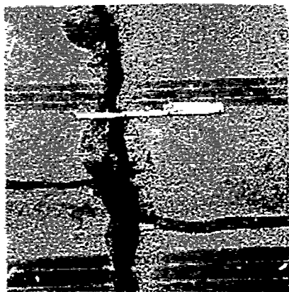
Photograph 15. Crack No. 6 on runway location before routing showing extent of previously applied sealing material.
