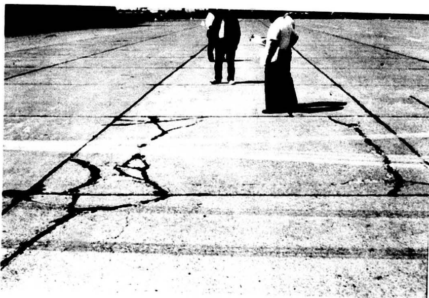
Figure 41. Severely Shattered Slab Located Along Traffic Line.
