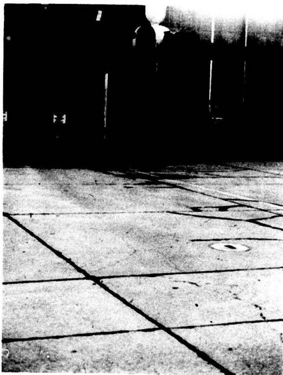
Figure 40. Pavement Damage Along Traffic Lines.
