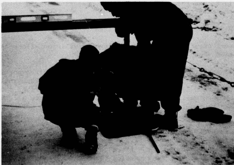
Figure 3.4.3. The expansion beam jacks should be about 1/2 in. above level or more to allow for settlement of the bearing surface.
